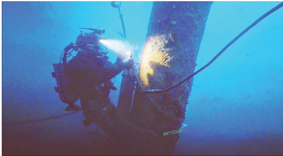
On Dec. 7, 2021, John Ditkof installs an anode — a component welded to underwater structures to prevent corrosion — in Akutan, Alaska.
