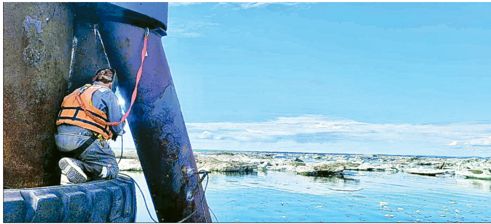
On July 2, 2023, John Ditkof repairs a mooring dolphin in the Port of Red Dog Mine, Alaska. Mooring dolphins are used to help secure a ship to a pier.
