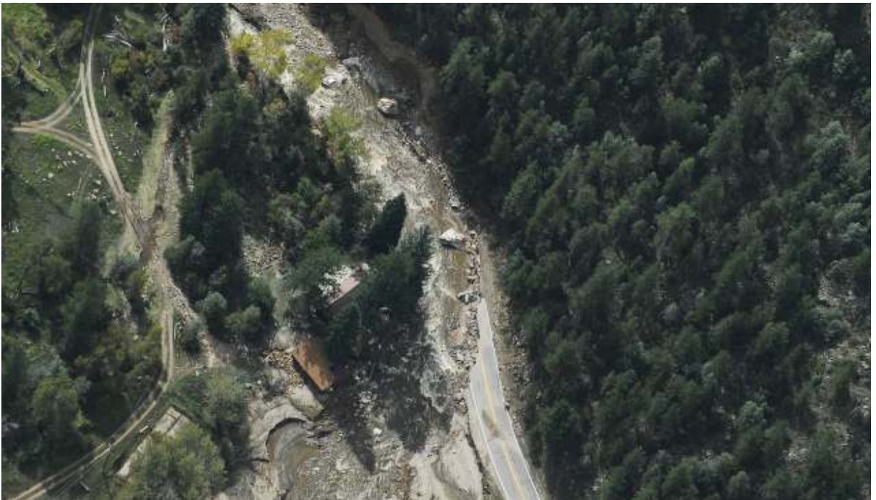
This aerial photo 1st Lt. Rob Pehkonen took near Estes Park, Colo., depicts just one of numerous areas where the highway was washed away. Though Colorado Gov. John Hickenlooper established a Dec. 1 deadline for certain bridges and roads to be repaired at least temporarily, the first snow of the season — in September, before CAP’s mission was concluded — was a reminder to residents that this winter could be particularly challenging.
