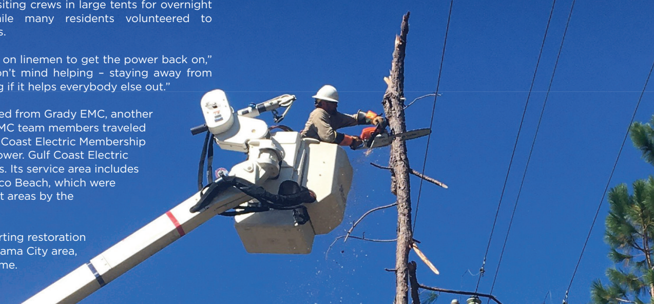
JACKSON EMC SENT MORE THAN 60 TEAM MEMBERS TO HELP RESTORE POWER IN GRADY COUNTY, GEORGIA FOLLOWING HURRICANE MICHAEL.
