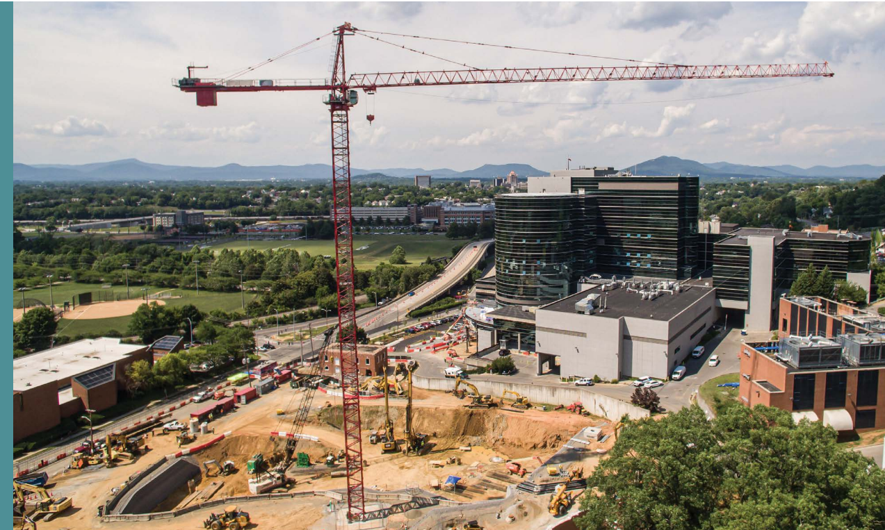
A 240-foot crane—the second tallest structure in Roanoke—was erected to help build our Crystal Spring Tower.
