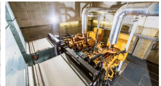
update energy supply airfield CHF ~15 million
