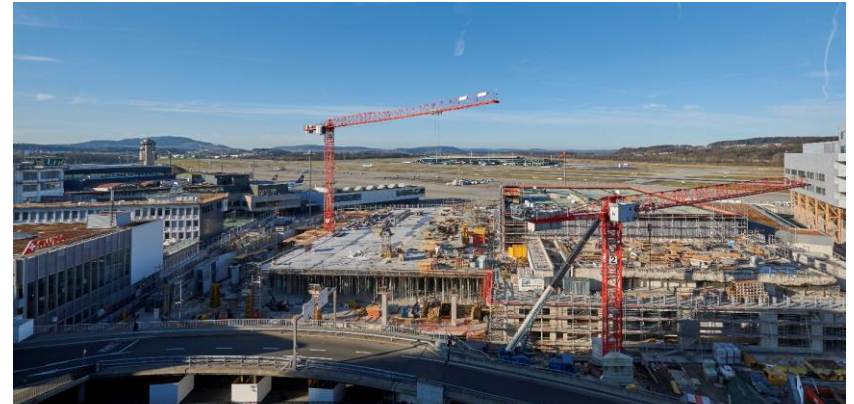
Baggage Handling System CHF ~50 million
