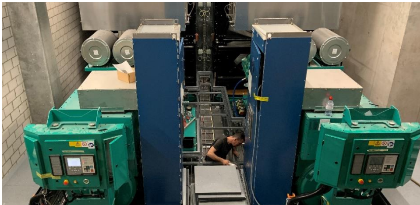
Upgrade Power Supply System CHF ~15 million
