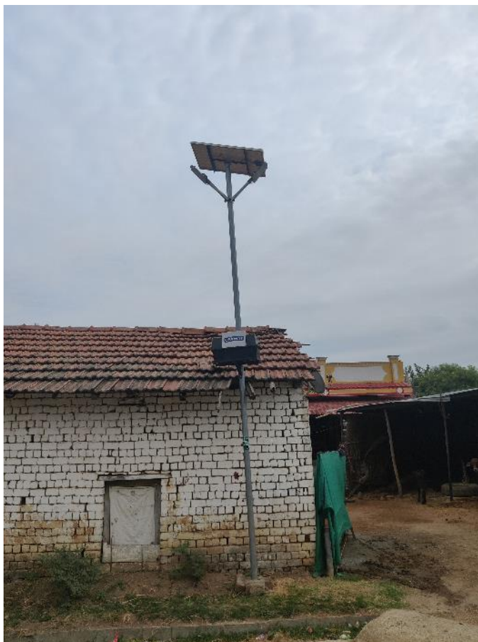
Street light installed by LT Foods in a village
