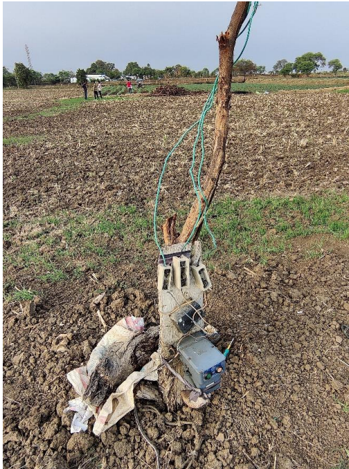
Electric motor used for extracting ground water
