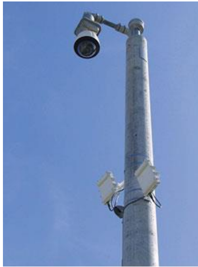
Figure 3. Typical Installation of a Pole-Mounted Traffic Camera (Source: Federal Highway Administration)
